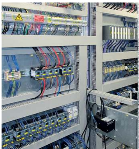
↑ High quality components in the electro-container
