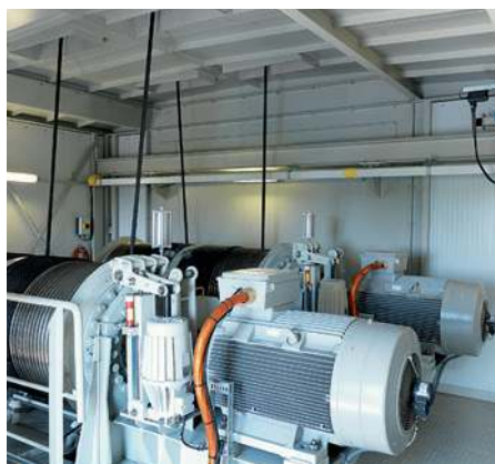
↑ Machinery room: spacious and maintenance-friendly
