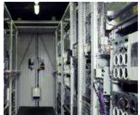
↑ Open electrical racks increasingly popular
