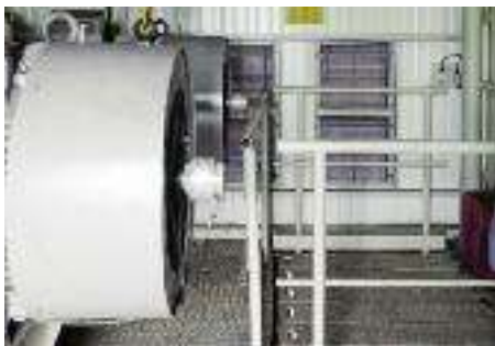
↑ The spacious machinery house allows for good reachability and easy maintenance
