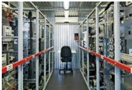
↑ Inside the electrocontainer
