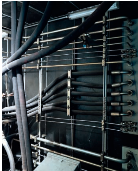
↑ Sound-insulated machinery room with clear layout
