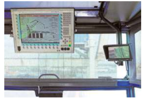
↑ Visualisation of crane data via Crane Management System
