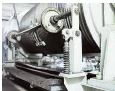
↑ Rope pressure device for safe hoisting rope winding
