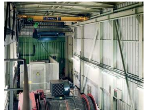
↑ Maintenance hoist inside of machinery house
