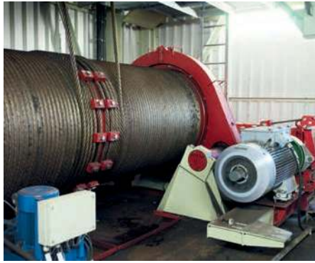
↑ Boom hoist system with safety band brake
