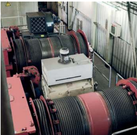
↑ Arrangement of hoisting and closing winch inside of machinery room
