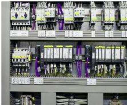
↑ View to cubicles on trolley
