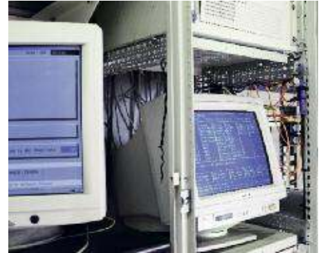
↑ Separate working station for engineers
