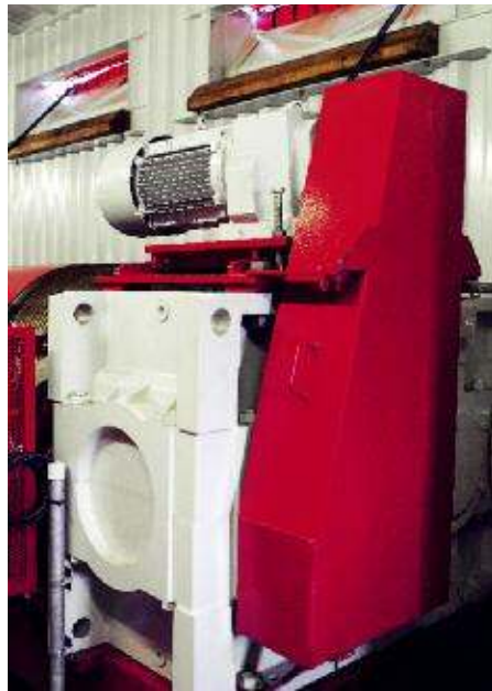
↑ Emergency drive for boom hoist
