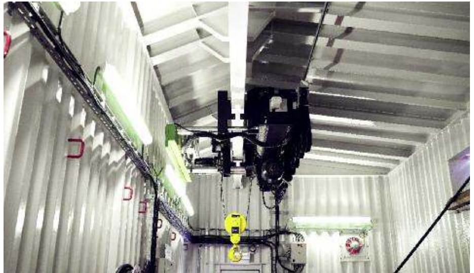
↑ Maintenance crane inside of machinery house
