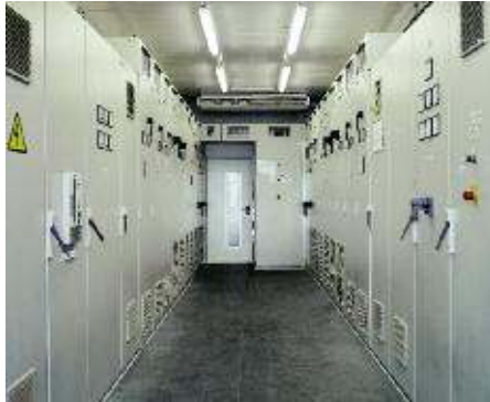
↑ Cubicles inside electrical house
