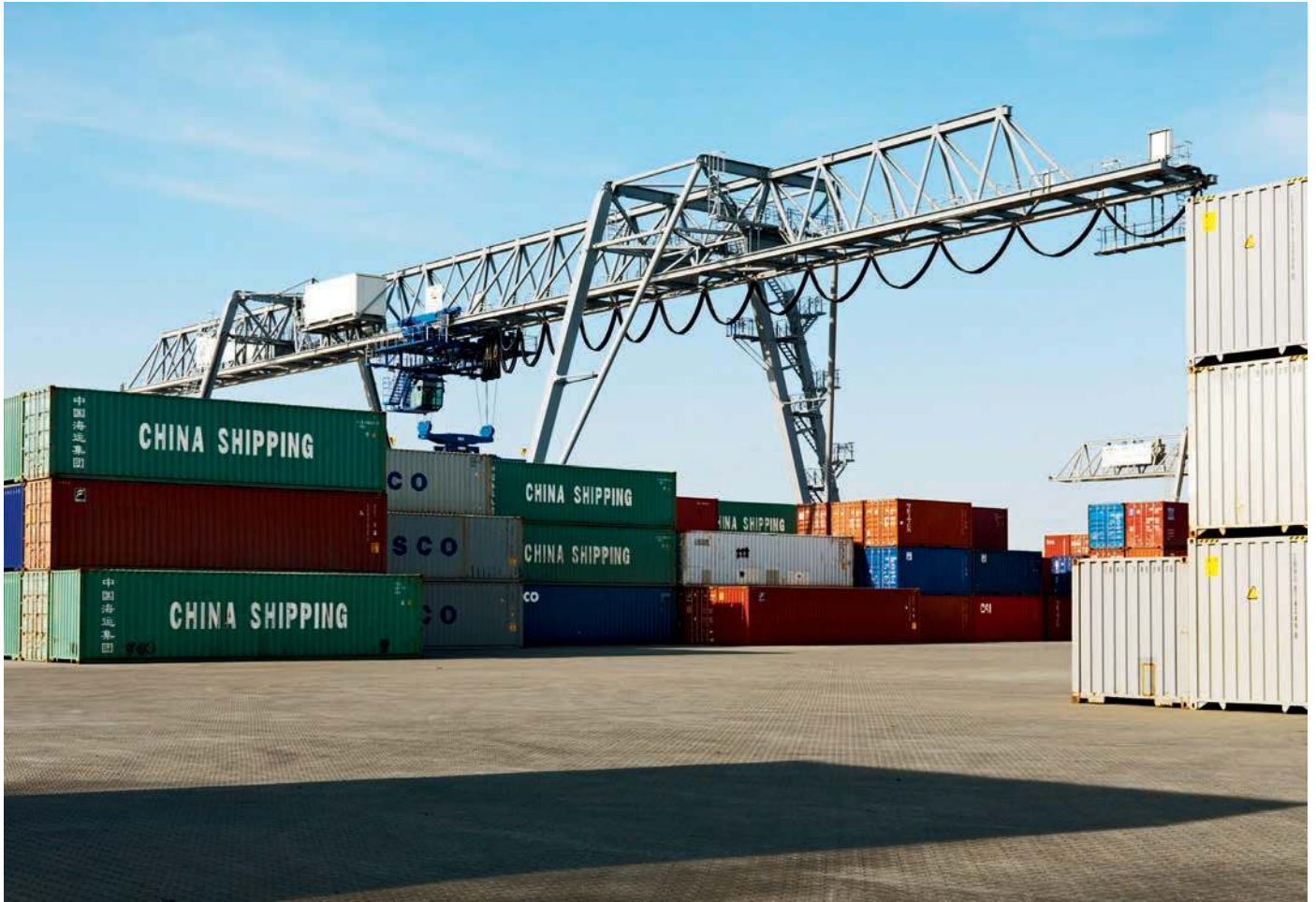
↑ Inclination of the gantry supports
