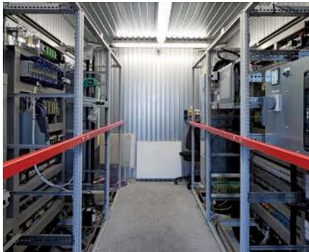
↑ Inside the electrocontainer
