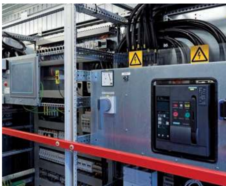
↑ Switch racks in the air conditioned electrocontainer
